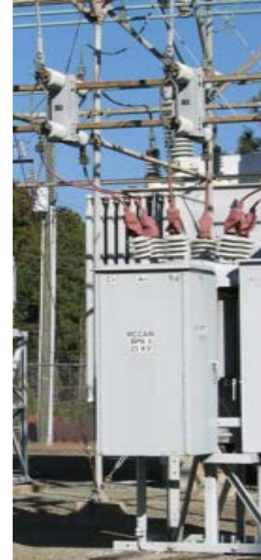
Substation Circuit Breaker
